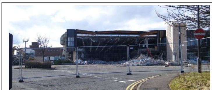
And now the end is near, as large demolition machines move in to destroy the physical plant where so much human creativity was unleashed.
